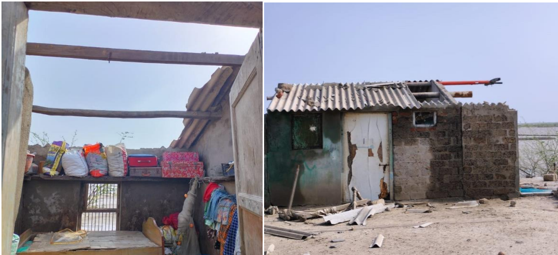
Pic 4 and 5: Damaged roof of the houses in Jangi Kantha Vistar
